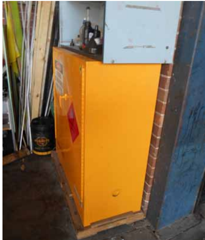
Photo 6 - Cabinet for fuel storage
