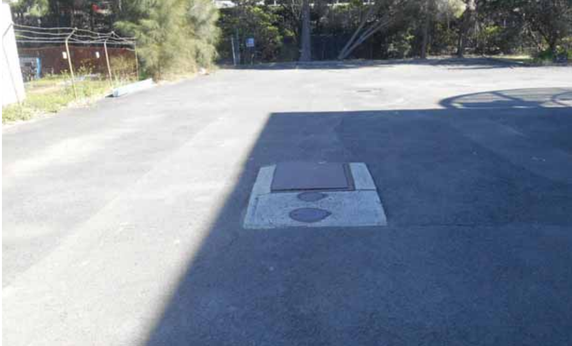
Photo 3 - Underground Storage Tank
