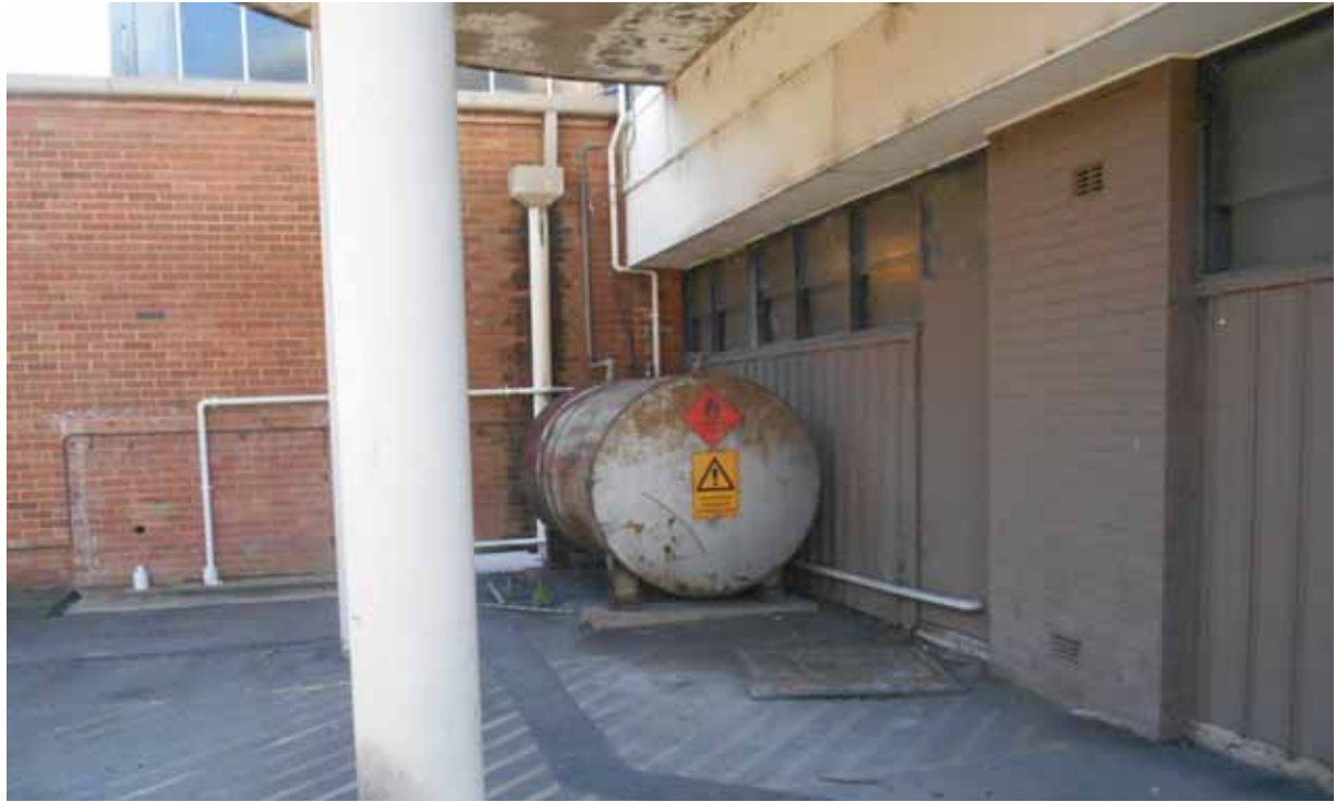
Photo 5 - Aboveground storage tank
